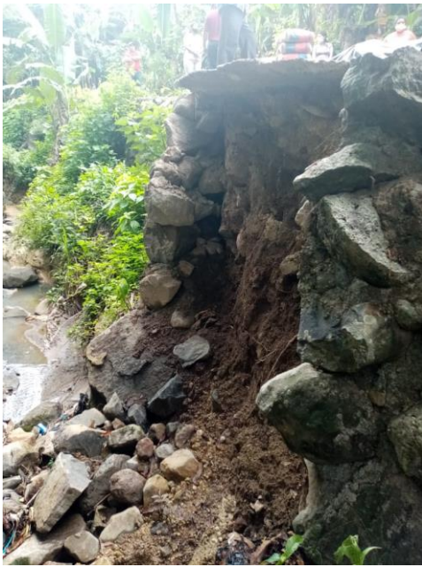
LANDSLIDE AT PANCHIMALCO
